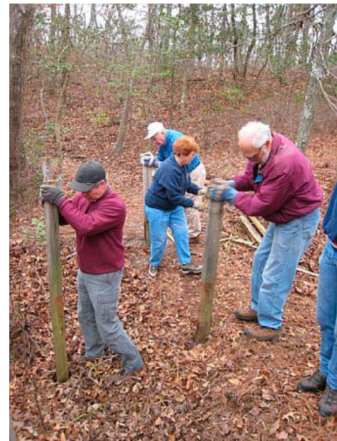
Tidewater Chapter members build a bridge on their adopted trail at First Landing State Park.
